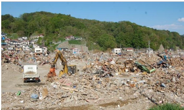
Efforts to remove the rubble at the Kuwagasaki area in Miyako City was progressing.
